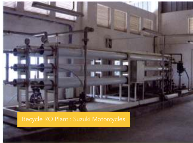
Recycle RO Plant : 660m 3 /hr. Oman
